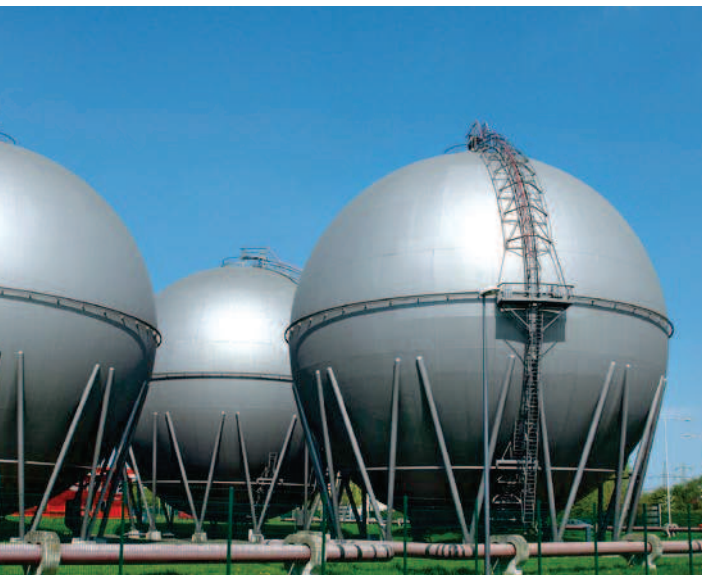
Odorizing of natural gas
