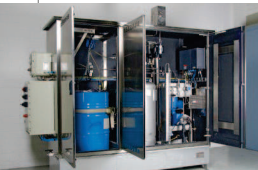
OD 240 in cabinet with heating unit and insulation, transfer from disposable drums, Ex controls suitable for hazardous areas.
